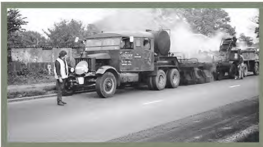
● Belonging to road-surfacing contractors W & J Glossop, this Pioneer is coupled to a specialised 'burner' trailer designed to strip the worn surface from the road, discharging it to an open truck by a loading elevator. The tractor is in surprisingly straight condition bearing in mind the work that it is undertaking.
